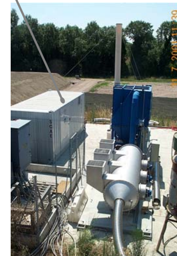
Gas- effluent treatment system
