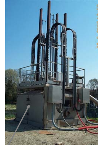
Gas- effluent capture system
