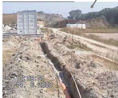
15 kV power line
